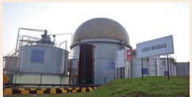
Biogas plant is a contributor to the source of electricity to the nation.
